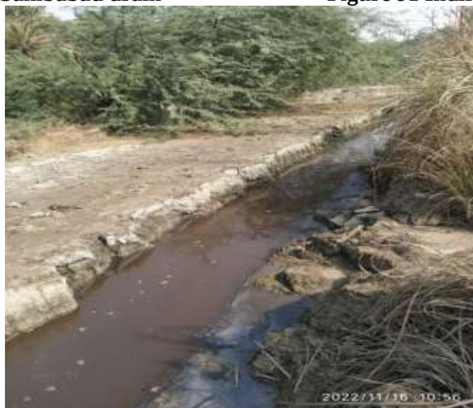
Figure 92 Banthala drain carrying industrial effluent
