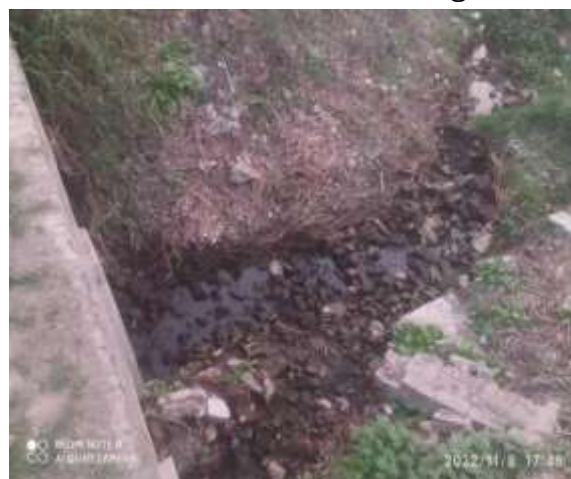
Figure 74 Kinauni Drain confluence with River Hindon
