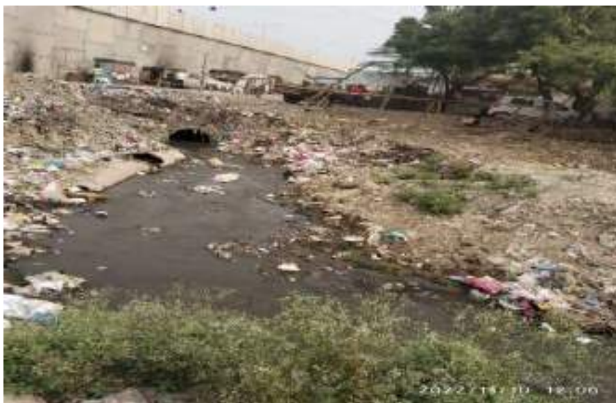
Figure 87 Rahul Vihar drain
